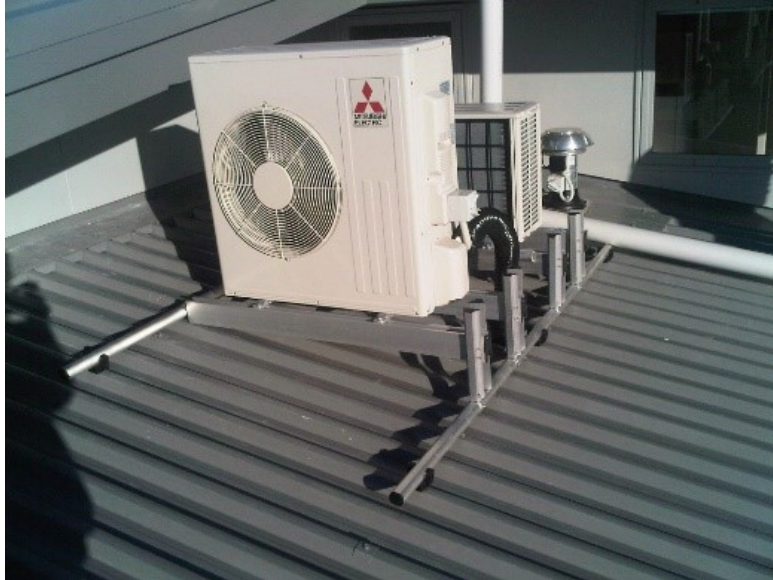
An air conditioning unit correctly installed on a roof, using durable and compatible materials.
